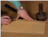
Lay out the same curve on a template. Take the beginning and ending points for the arc from the drawings, then connect the points using the same batten technique.
